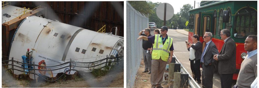
Council Members (from center) John Schmidt , Jeff Wilhite and David Hamilton, learn about the Canal Interceptor Tunnel at the Hickory Street Ohio Canal Interceptor Tunnel 1 site where "Rosie" the Tunnel Boring Machine is located .
